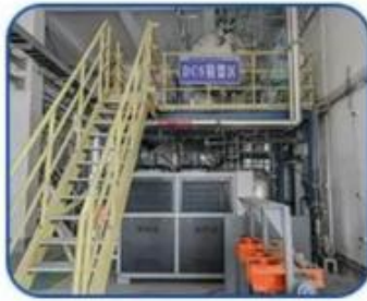
Zone of rectification
